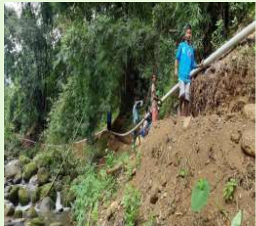
Pipe Line from Source to Village
