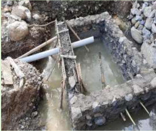
Siltation Tank at source
